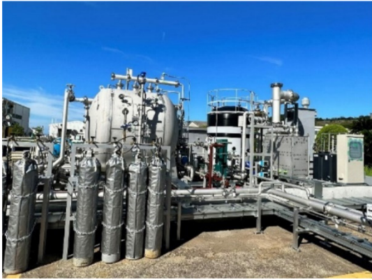
Figure 9 Ammonia handling demonstration test facility
