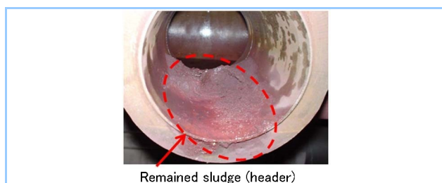
Figure 8 Residual sludge of once-through boiler after chemical cleaning (organic acid is applied)
