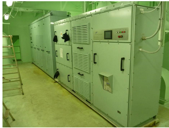
Figure 3 External view of inverter (left) and converter (right)
