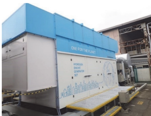
Figure 6 Hydrogen engine generation set
