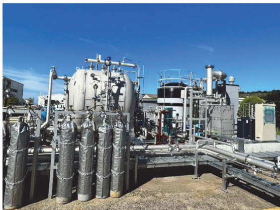
Figure 1 AGAS demonstration facility
