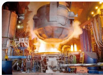
Large Electric Furnace (EAF Ultimate)
