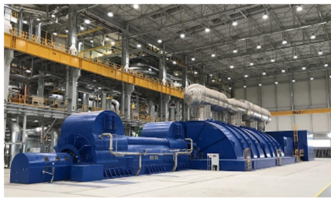
Figure 9 Poland Kozienice power plant No. 11 unit
