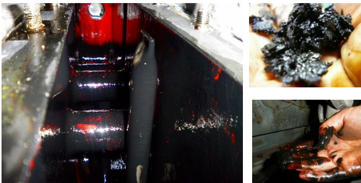
Accumulated sludge at the bottom of the tank
