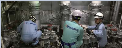
Modifying control system devices
