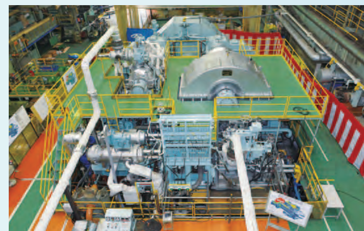
UST (Ultra Steam Turbine)
