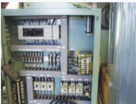
Sequencer (controller) within the control panel
