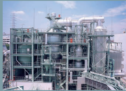
Sewage Sludge Treatment Plant
