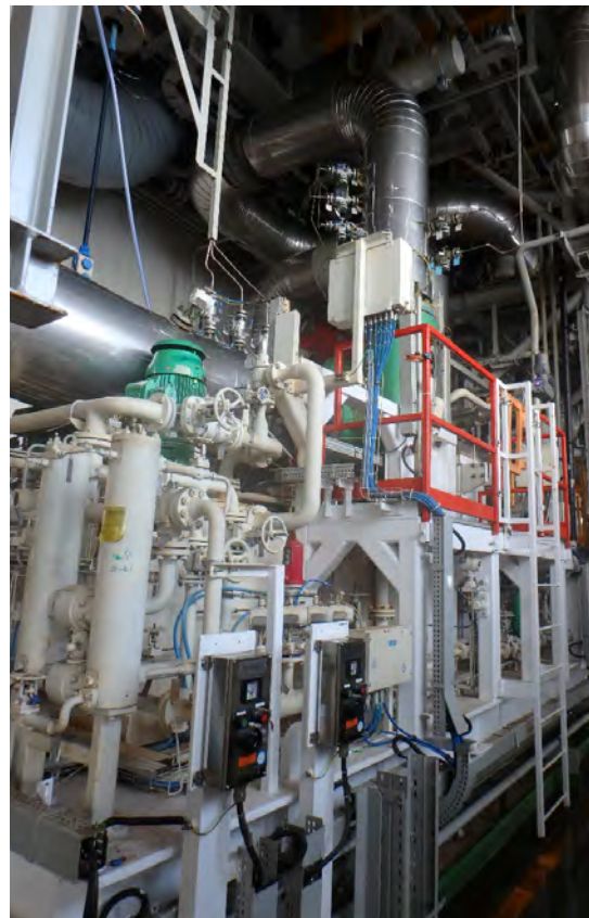
Several Rotoflow compander models have been marinated or specifically tailored for coastal or offshore applications, as seen in this FLNG facility, to withstand the harsh and corrosive saltwater environment. Courtesy of Rotoflow.
