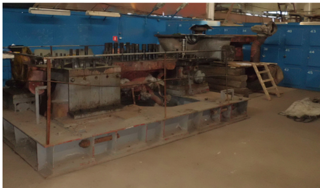
Figure 1. The existing syngas turbine casing in a customer's plant (Russia) before modernisation.
