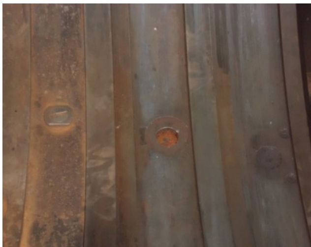
Figure 2. Additional unknown screw inside turbine casing.
