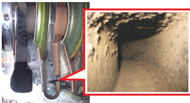
Figure 4. A rough surface inside a compressor due to fouling
