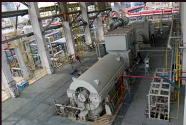
Elliott compressor installed in a PDH application in China.
