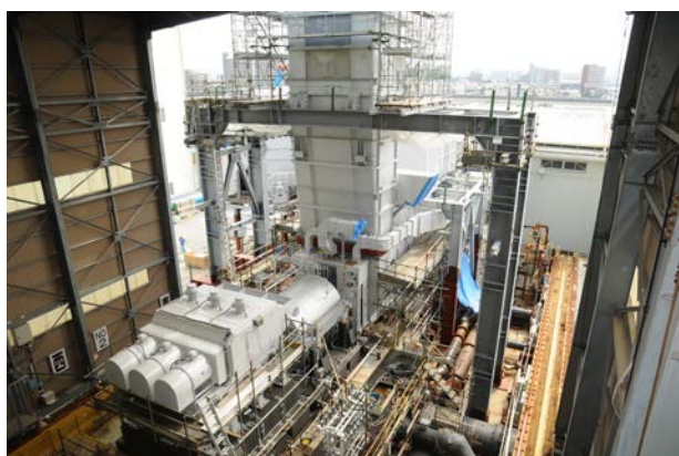
Figure 2. MR LP compressor – gas turbine string on test stand in Indonesia.
