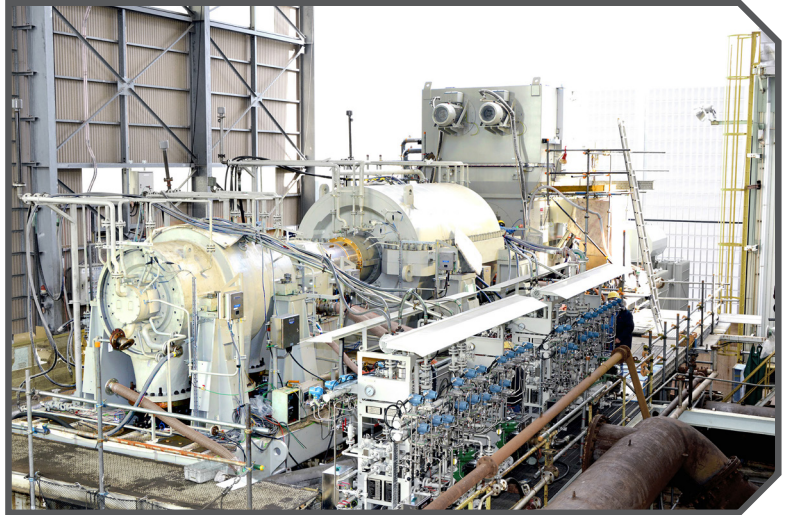
Mitsubishi Heavy Industries Compressor International: MHI LNG refrigeration compressor train.
