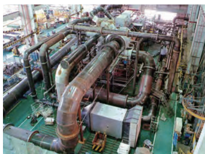
Integally Geared Compressor for PTA Plant
