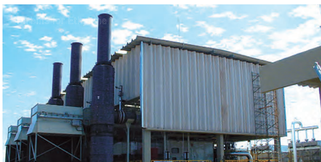
Gas Pipeline Station
