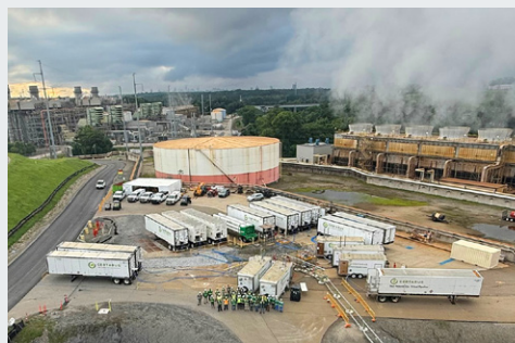
Plant McDonough-Atkinson (photo courtesy of Georgia Power)
