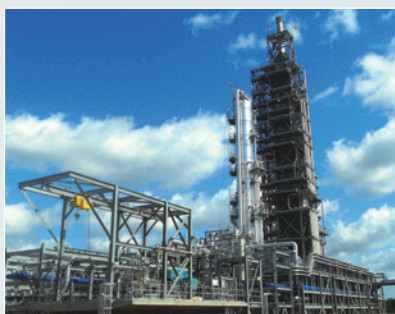
CO 2 capture plant
