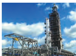
CO 2 capture plant
