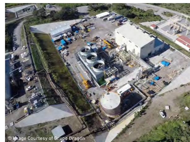
© Image Courtesy of Grupo Dragón Geothermal generation facility (Mexico)
