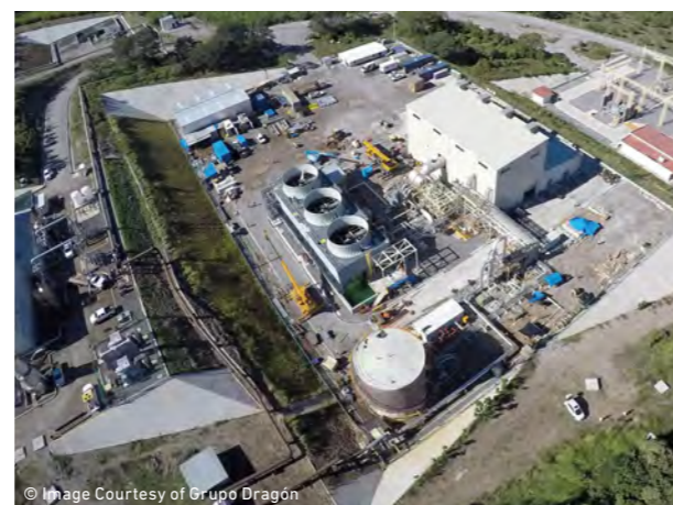
Geothermal generation facility (Mexico)
