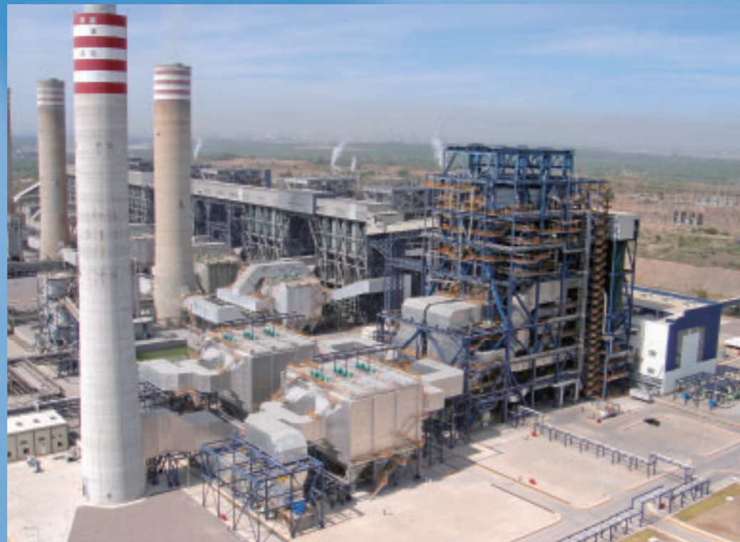
New Pacifico power station fronts six power stations that also feature MHI products, together accounting for 43% of the thermal power generation capacity in Mexico.
