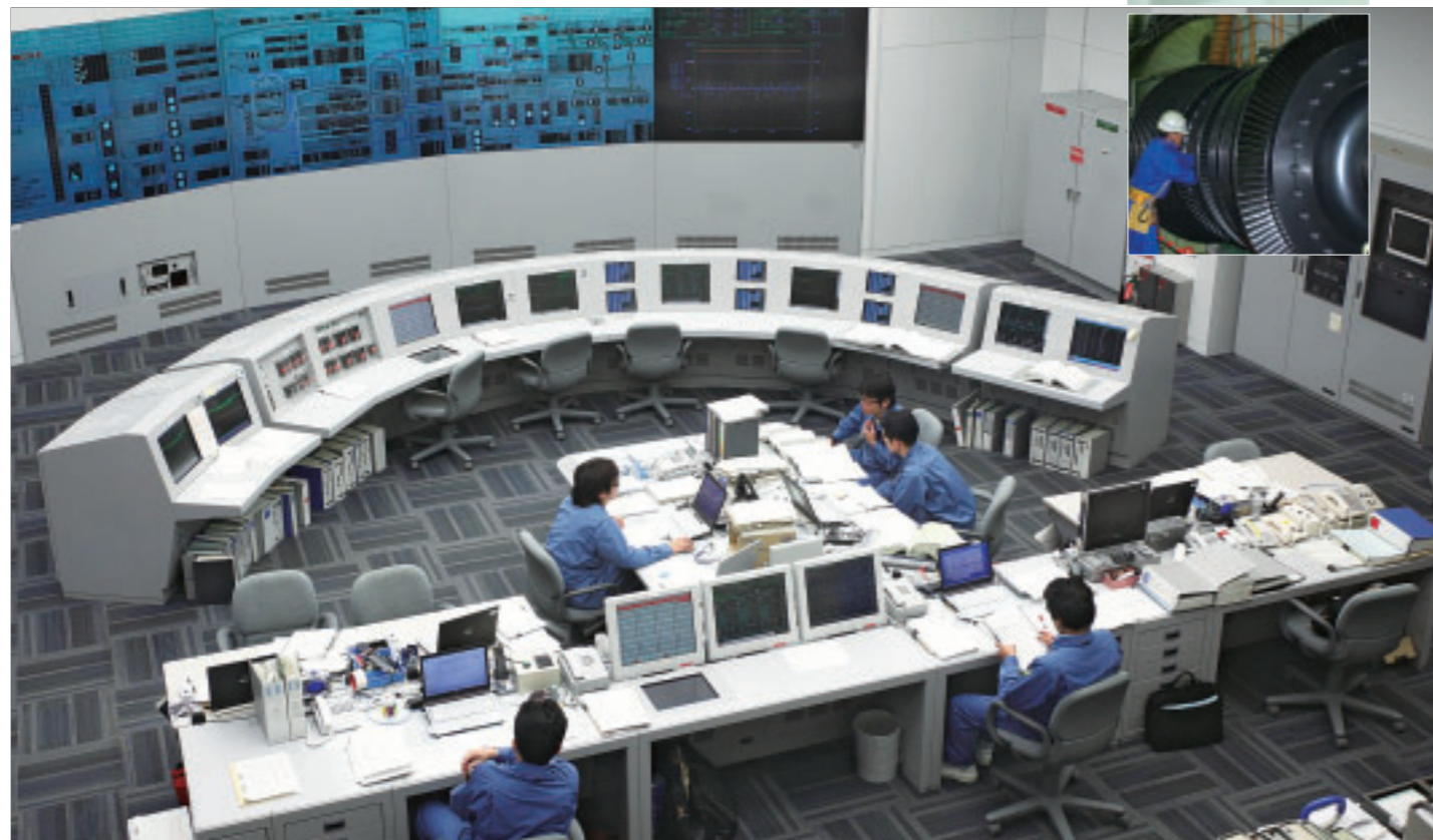
(Bottom) The central control room where all equipment, including the nuclear reactor, turbines and power generators, are operated, monitored, and controlled. (Right) Turbine inspections involve meticulous checking down to the fine details.
