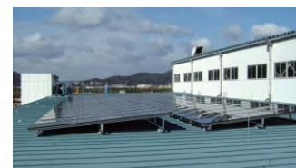
Solar cell panels installed in the Paper & Printing Machinery Division
