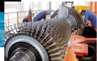
Supplying GTCC technology in China to realize higher power-generating efficiency and reduce environmental loads amid a steady rise in power demand
