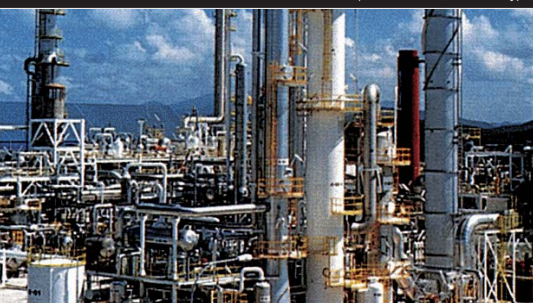
CO 2 recovery plant
