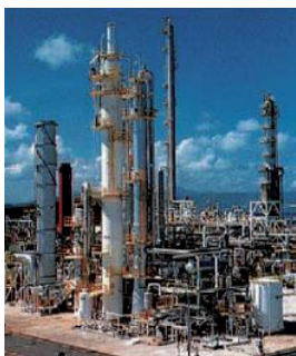
CO 2 recovery plant
