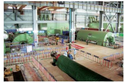
Huizhou Power Plant
