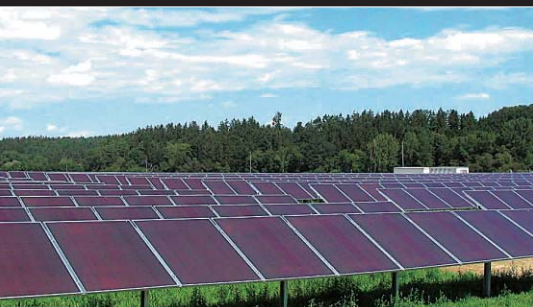
Solar farm (near Munich, Germany)
