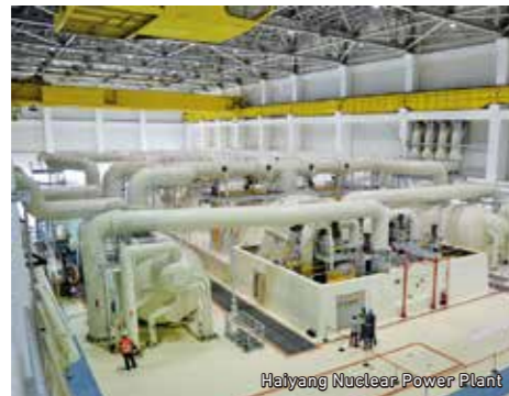
Nuclear Power Turbine Generation Equipment
