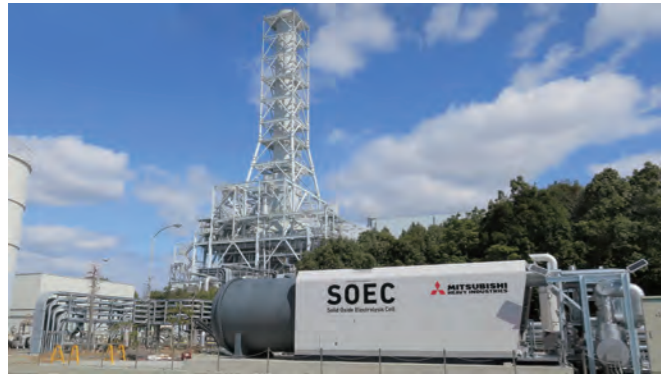
Figure 26 SOEC (Takasago Hydrogen Park)
