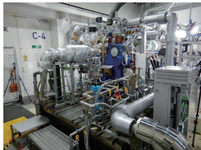
Figure 8 A hydrogen engine installed at the AIST Fukushima Renewable Energy Laboratory
