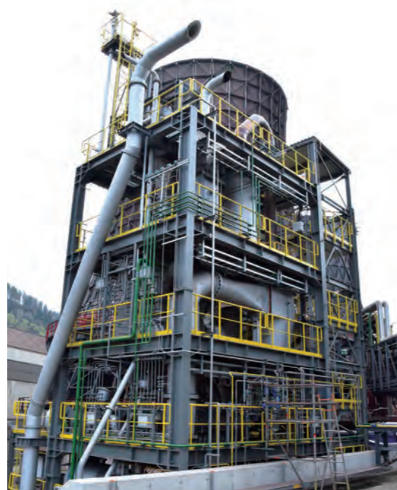
Figure 32 Hydrogen-based fine ore direct reduction (HYFOR) pilot plant
