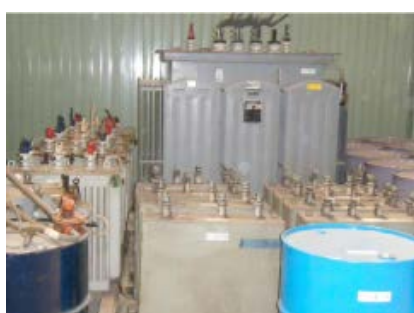
PCBs storage facilities at the Nagasaki Shipyard & Machinery Works
