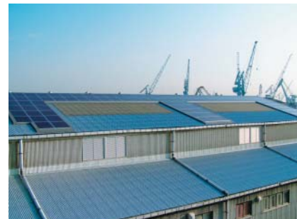
10 kW solar system installed at the Yokohama R&D Center
