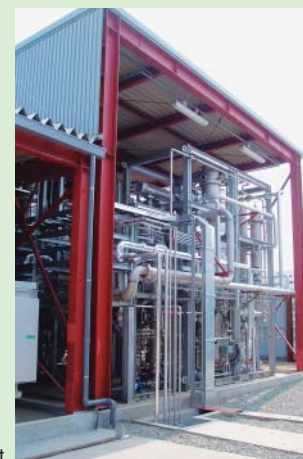
Solvent refining unit
