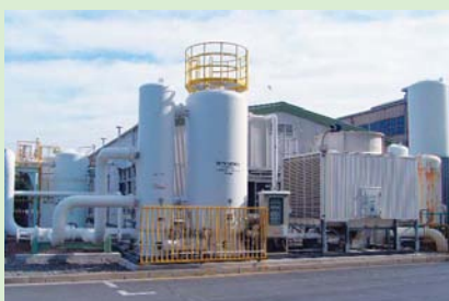
Equipment for removing moisture and oil, with compressed air heater
