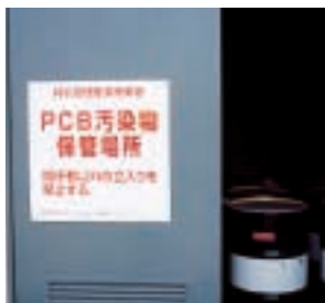
Checking storage condition of PCB
