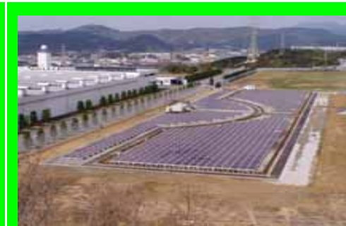
Solar power generation system
