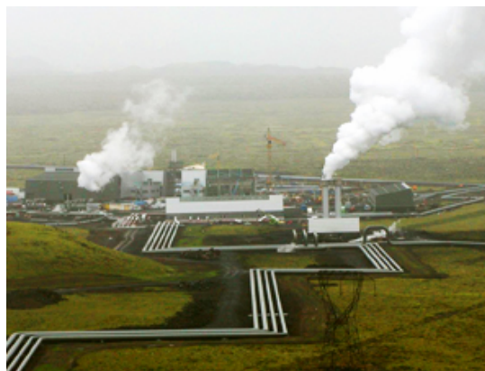
Iceland Nos. 3 and 4 units of Hellisheidi Power Plant
