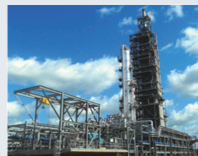
CO 2 capture plant
