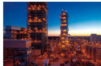
CO 2 capture plant (world's largest CO 2 capture volume of 4,776 tons / day for a power plant application)
