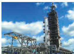
CO 2 capture plant
