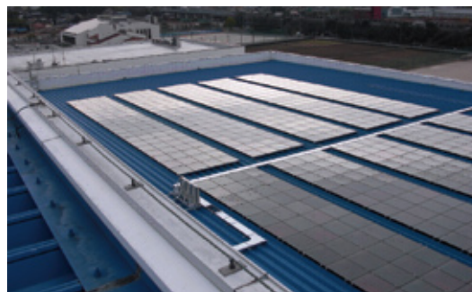
Solar cell panels at the Nagoya Guidance & Propulsion Systems Works
