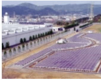
Photovoltaic Power Generation System
