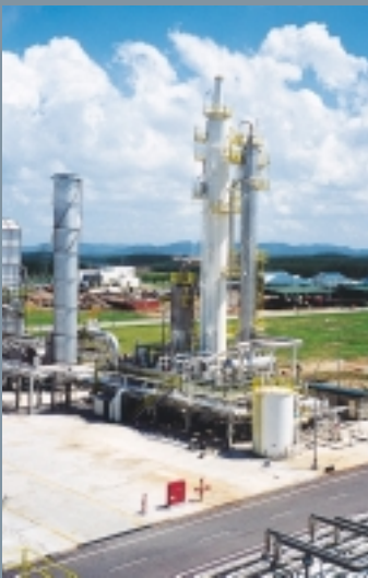
CO 2 Recovery Plant (Malaysia)
