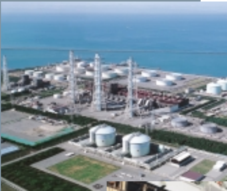
Unit No.4-1 Higashi Niigata Combined-Cycle Power Station of Tohoku Electric Power Co., Inc.
