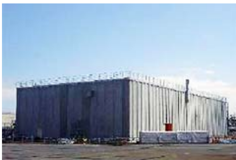
G2 Area sludge storage tank equipment at TEPCO's Fukushima Daiichi Nuclear Power Station
