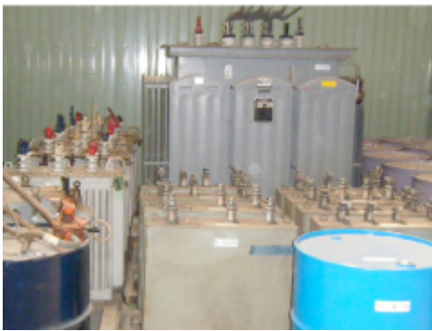
PCBs storage facilities at the Nagasaki Shipyard & Machinery Works
