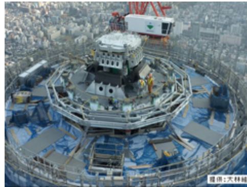
Tuned Mass Damper (TMD) vibration control system
