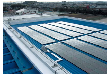
Solar cell panels installed at the Nagoya Guidance & Propulsion Systems Works
