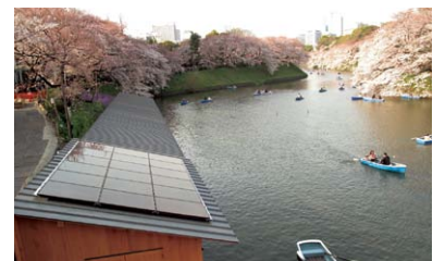
Photovoltaic facility installed on a boathouse roof
