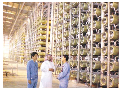
Inside a desalination plant
