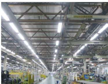
Plant lighting at the General Machinery & Special Vehicle Headquarters
