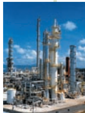
Flue gas CO 2 recovery plant
