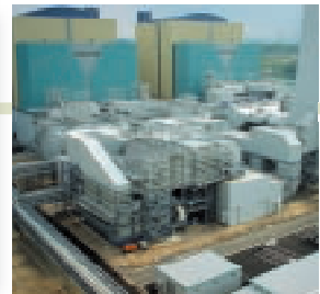
Flue gas desulfurization system
