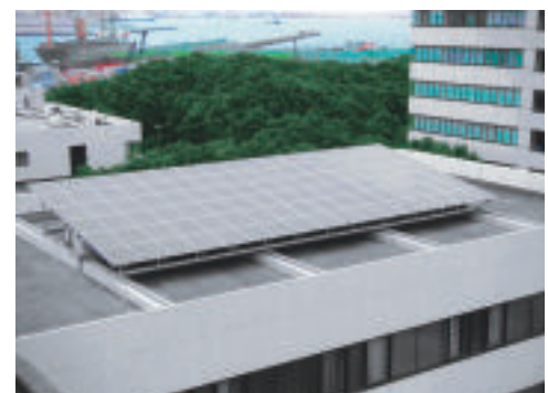
10 kW solar system installed at the Advanced Technology Research Center
