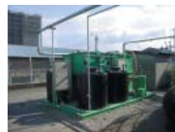
The purification plant which started operation
