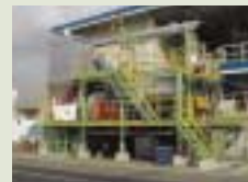
Sludge carbonizing oven
