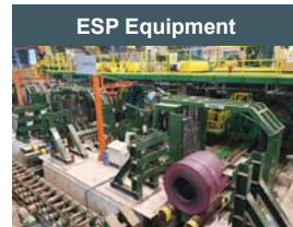
ESP Equipment Rizhao Steel (China) launches its fifth ESP plant with equipment supplied by Primetals
