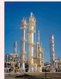
CO 2 capture plant
